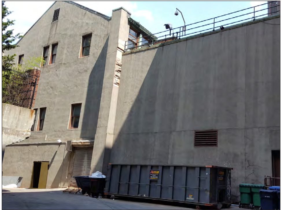
View east of Building 15, Building 15A, and a portion of the Museum's service yard 9
